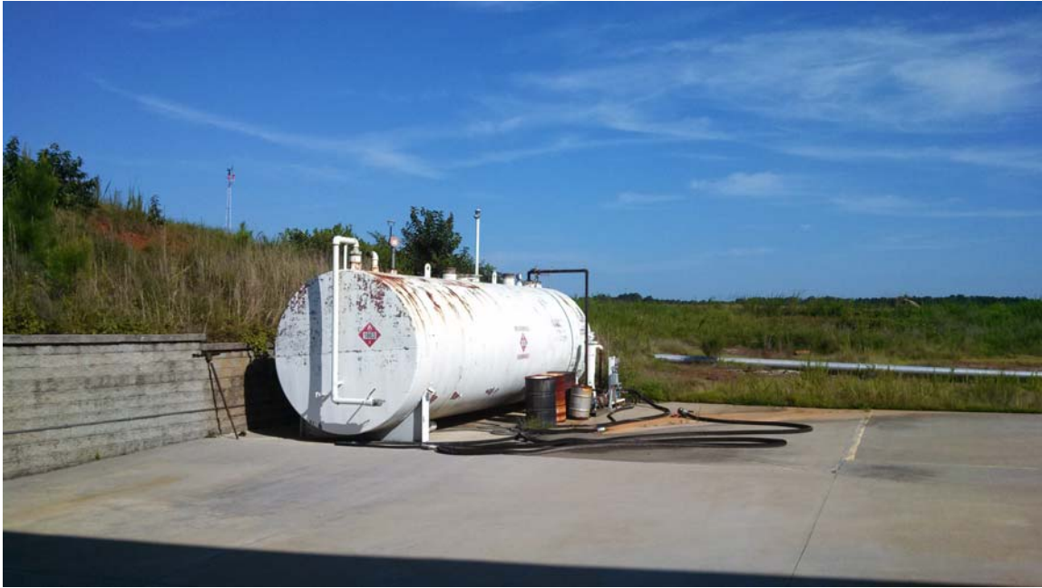
Onsite Fuel Storage
