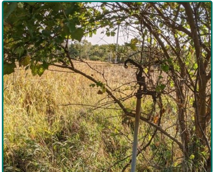
Well spigot next to electrical service and well
