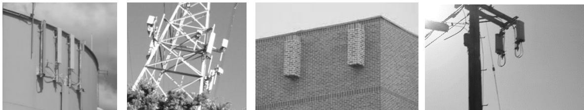
Examples of Flush Mounted Wireless Communication Facilities
