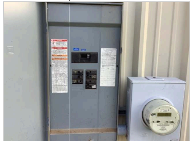
Garage wall entrance panel
