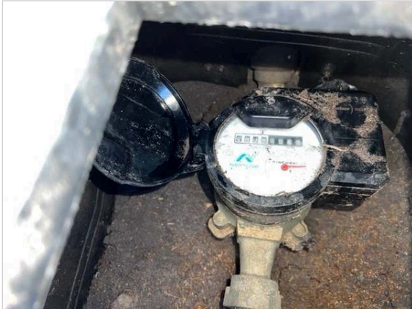
Water meter checked
