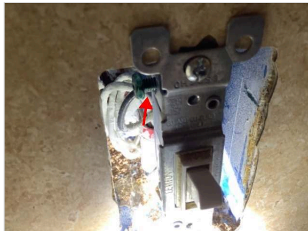
No ground wire
