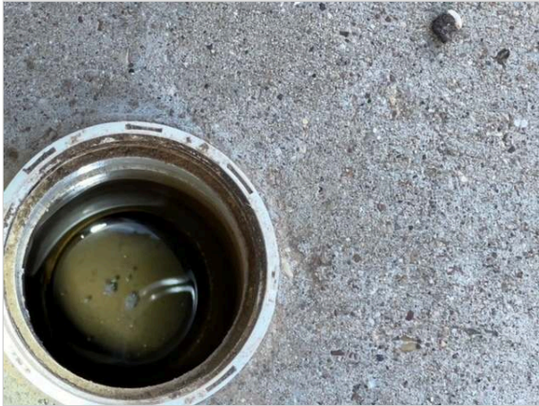
Water in cleanout
