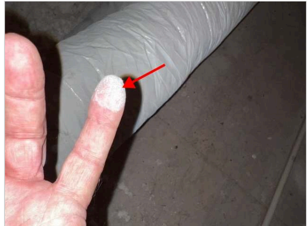
Residue in attic
