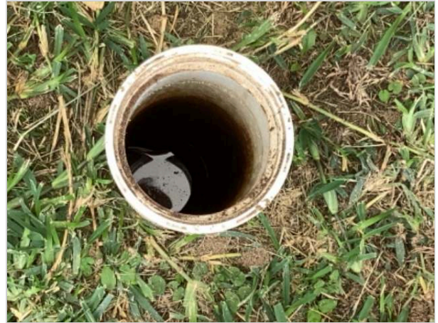
Water in cleanout
