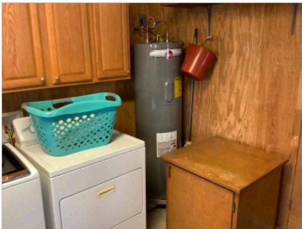
Garage water heater
