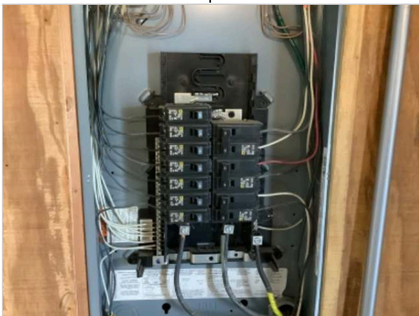
Garage sub panel
