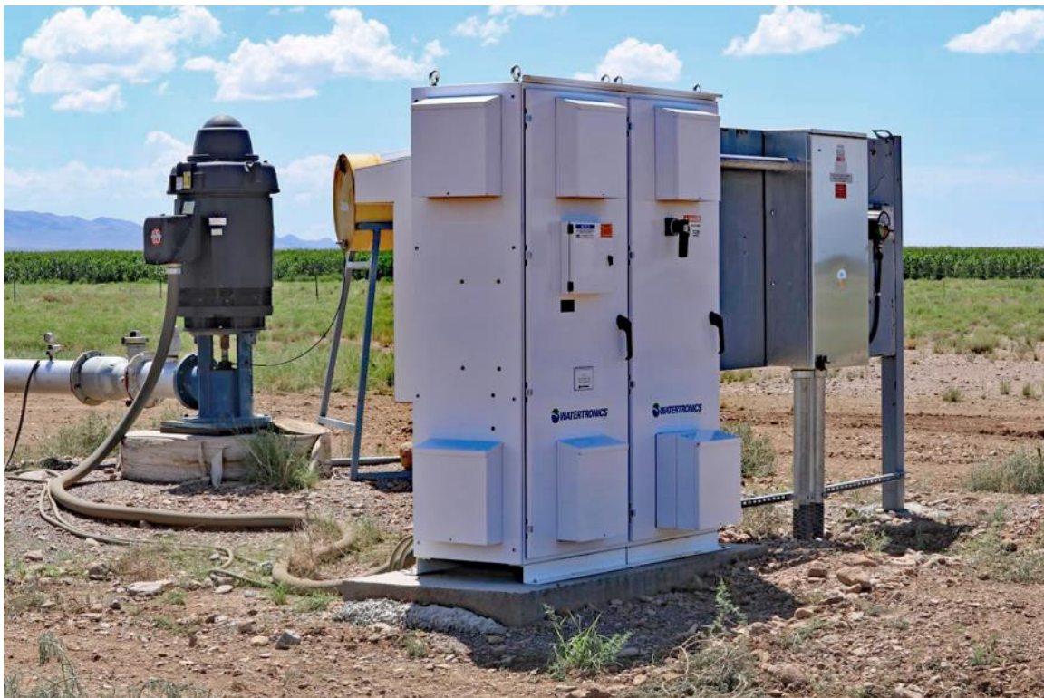
Well No. 1, drilled 2/24/20, 1090' deep, 250 hp, 1,000 GPM
