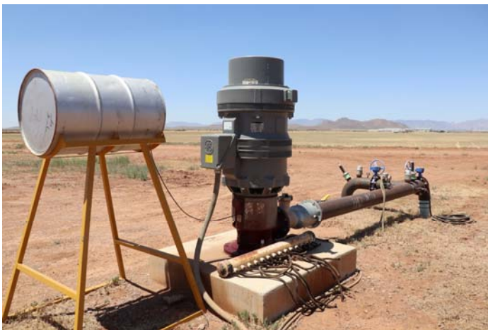
Irrigation well 500' deep, 150 HP, 675 GPM
