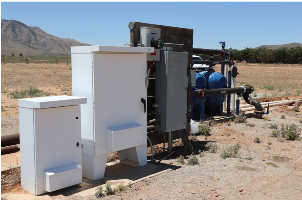
Well 915' deep with submersible pump, 250 gpm
