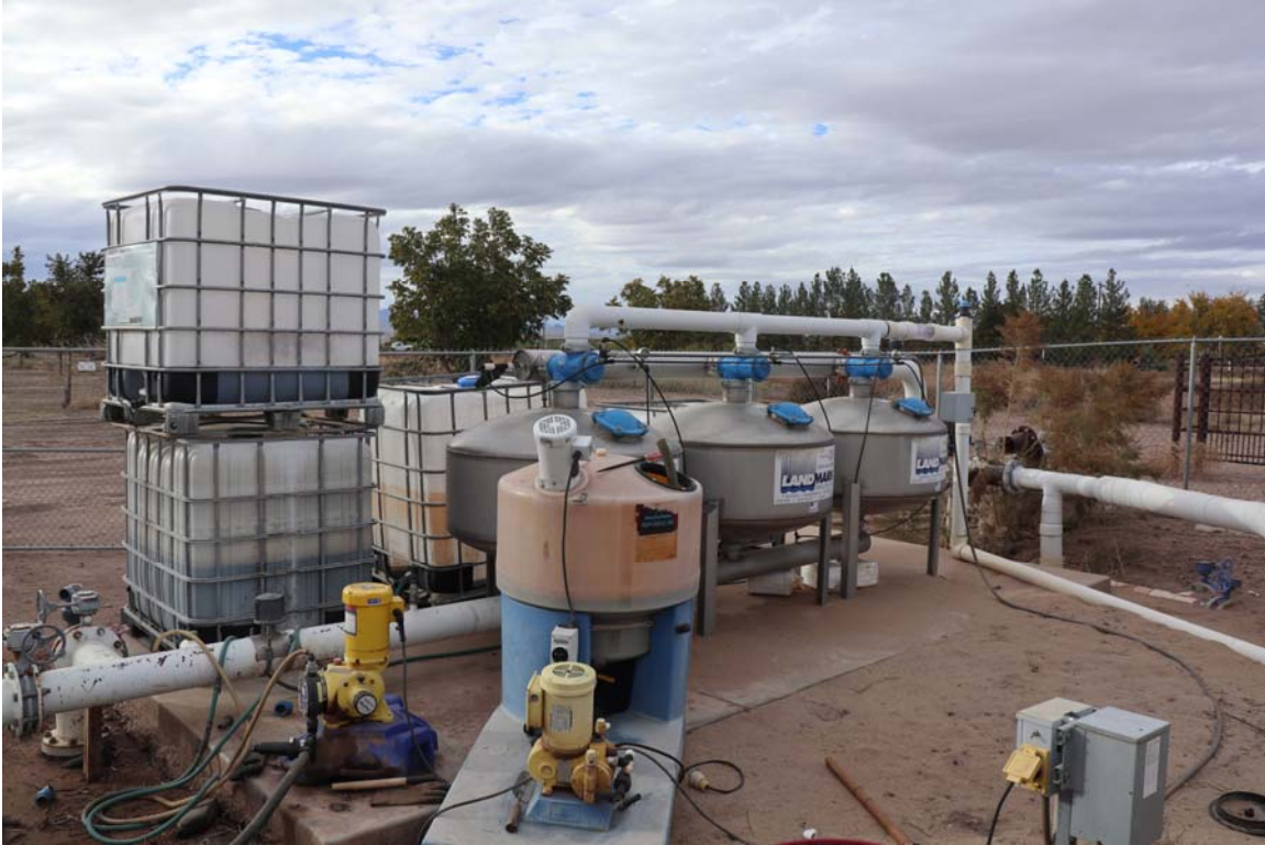
Flow Guard sand media filtration system
