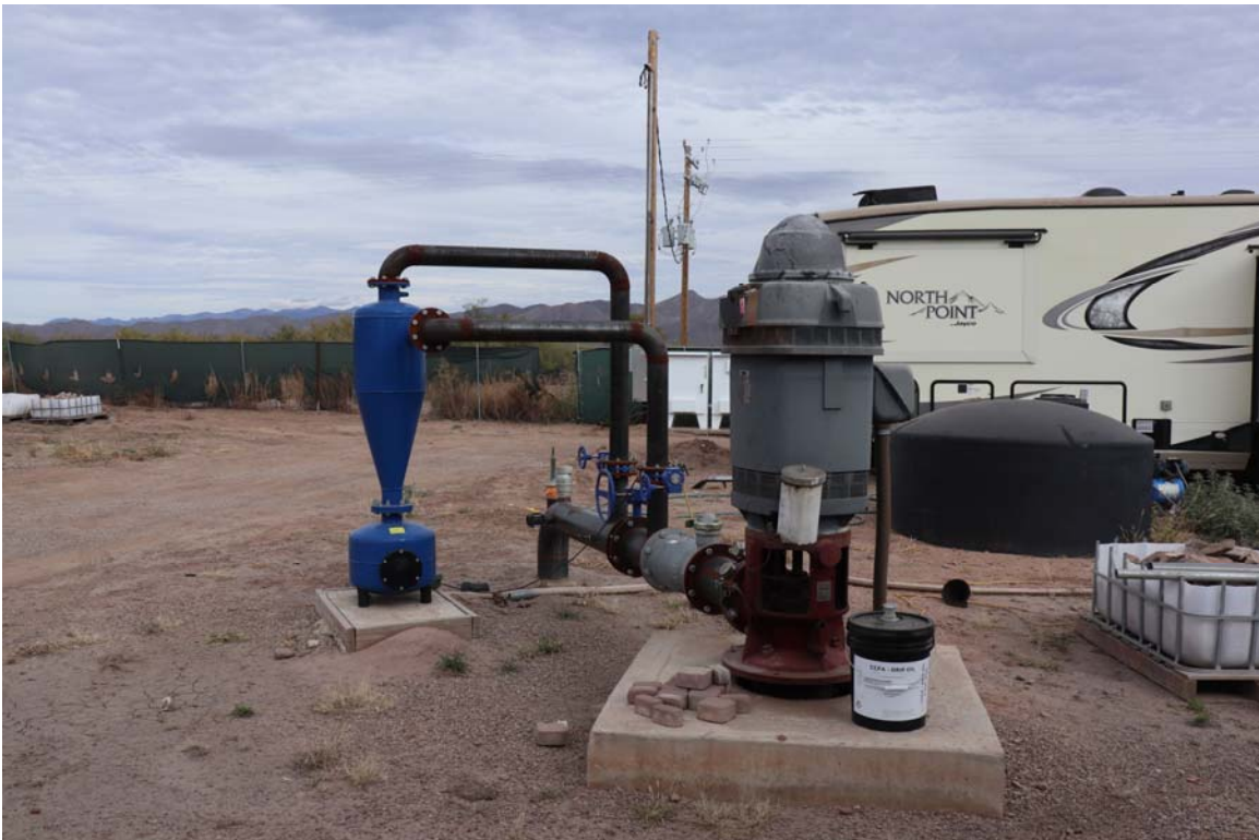
Well 1,005' deep, 12-3/4" casing, 150 hp, 600-650 gpm
