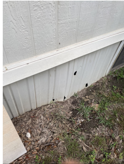
more damaged skirting
