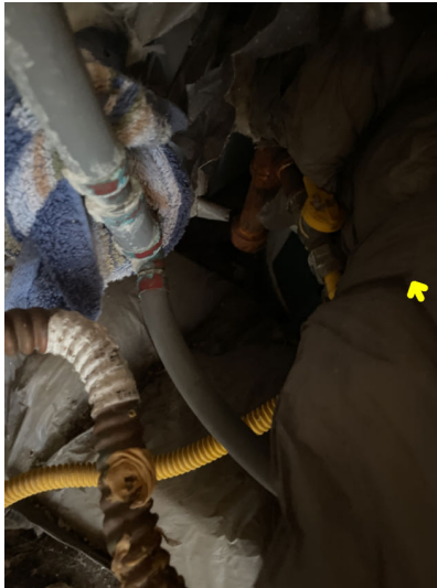
Gas valve for water heater
