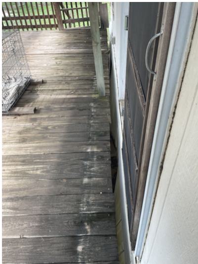
Recommend removing or completely overhauling this detached deck at the sliding door exit
