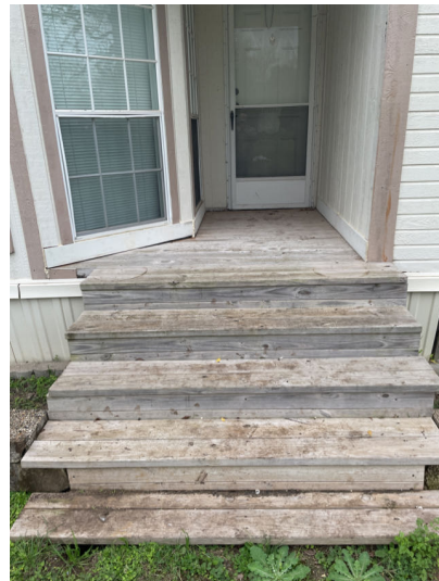
Railing should be installed for these steps
