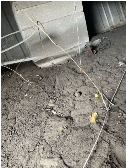
Loose Tie down/Anchoring system
