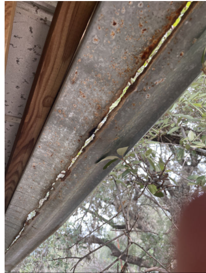
rusted through gutter on the deck area recommend removing and replacing
