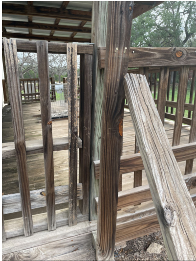
Hand rail not attached
