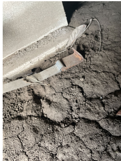
loose Tie down/anchoring system
