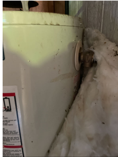
TP&R valve not piped down properly
