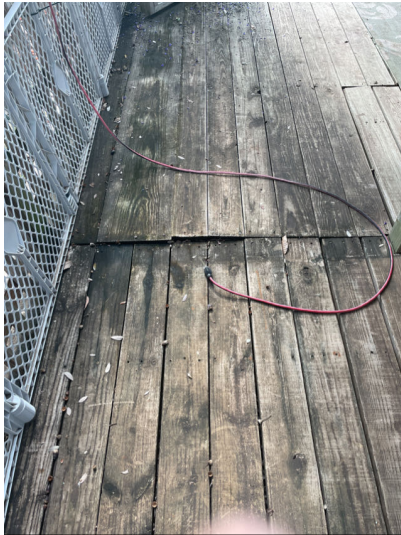
trip hazard on deck
