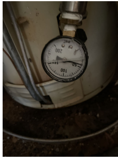
water pressure aprox 45 psi
