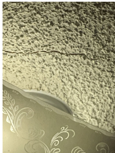
crack in ceiling
