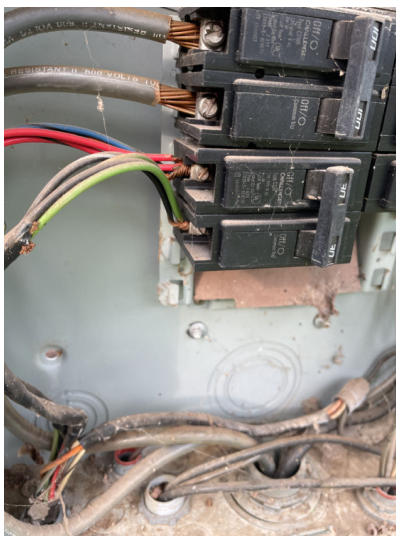
multiple wires lugged in one breaker
