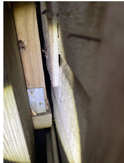
Deck appears to be toe-nailed to the home
