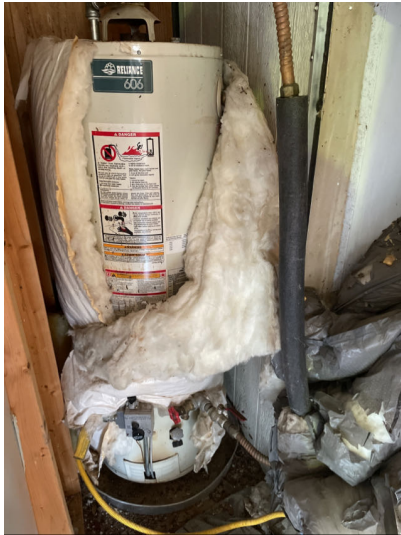
Water heater on deck
