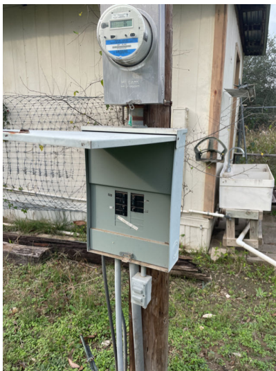
main service panel
