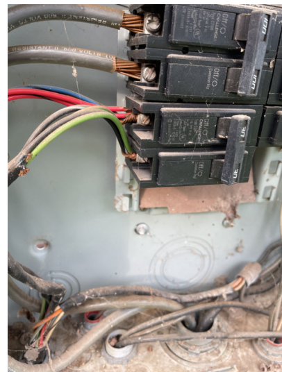
multiple wires lugged in one breaker
