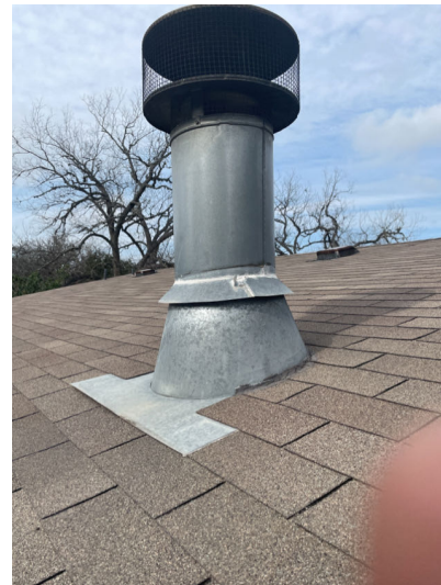
chimney appears to need the caulking redone
