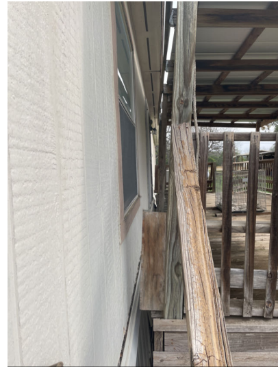
stand-alone deck appears to be falling away from the home
