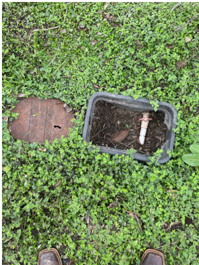
main water shutoff valve next to meter
