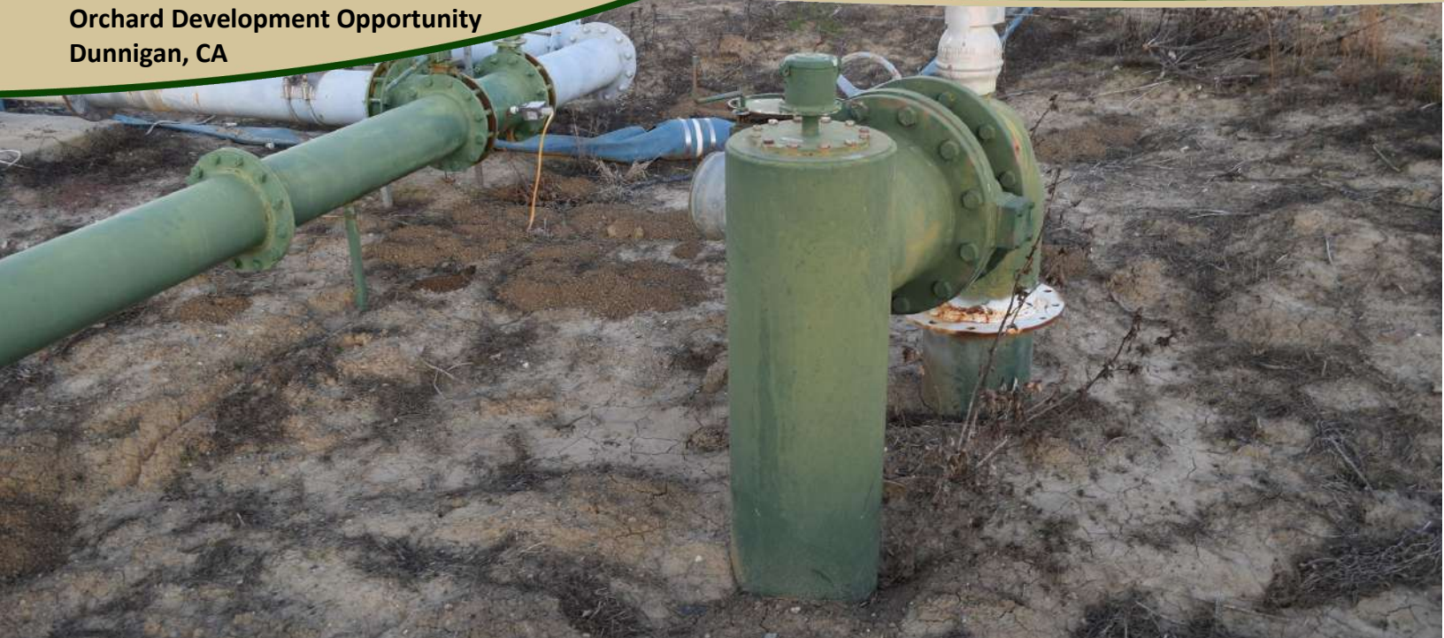
District Outlet#1 (DO#1)
